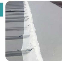
• The overlap between the light steel roof color steel plate and the daylighting board and the sealing of the joint of the gutter.
